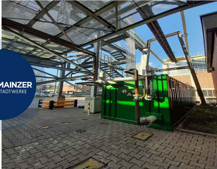
Mixing Station provided by Mainzer Stadtwerke
