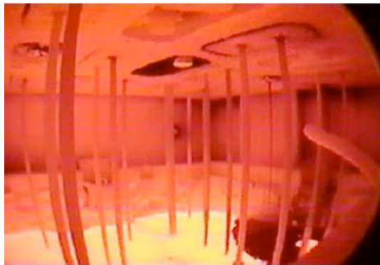
View inside JHCM plenum
