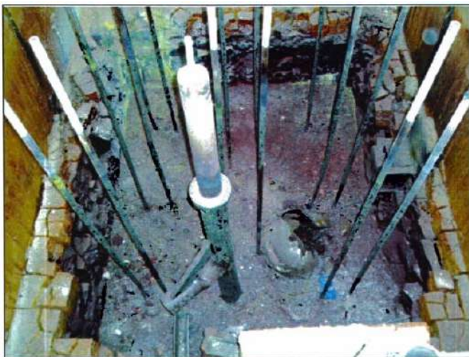
Inside view of DM3300 melter after its lid was removed. \text{SO}_4^{2-} rich yellow salt can be seen sticking to the refractory walls.
