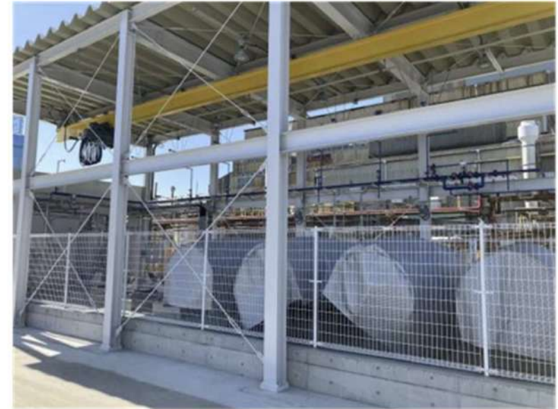
Storage tank for ammonia fuel
